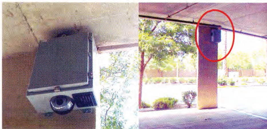
Security cameras that are exposed to the elements should be housed in weatherproof (and sometimes bulletproof) enclosures.
